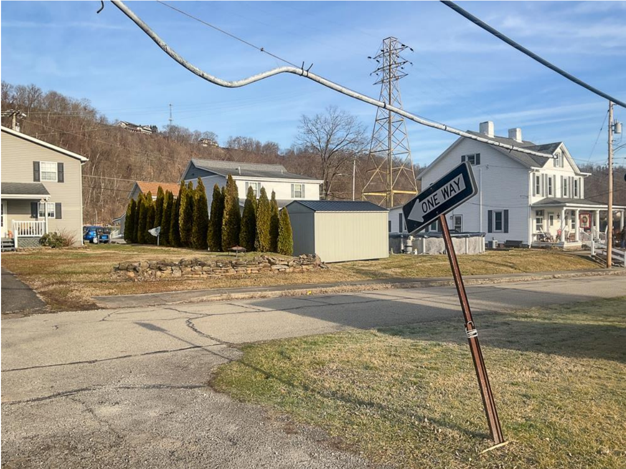
Lead cable sags between utility poles in Pennsylvania neighborhood Photo: Monique Rydel-Fortner
