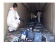
Disposal of lead acid batteries
