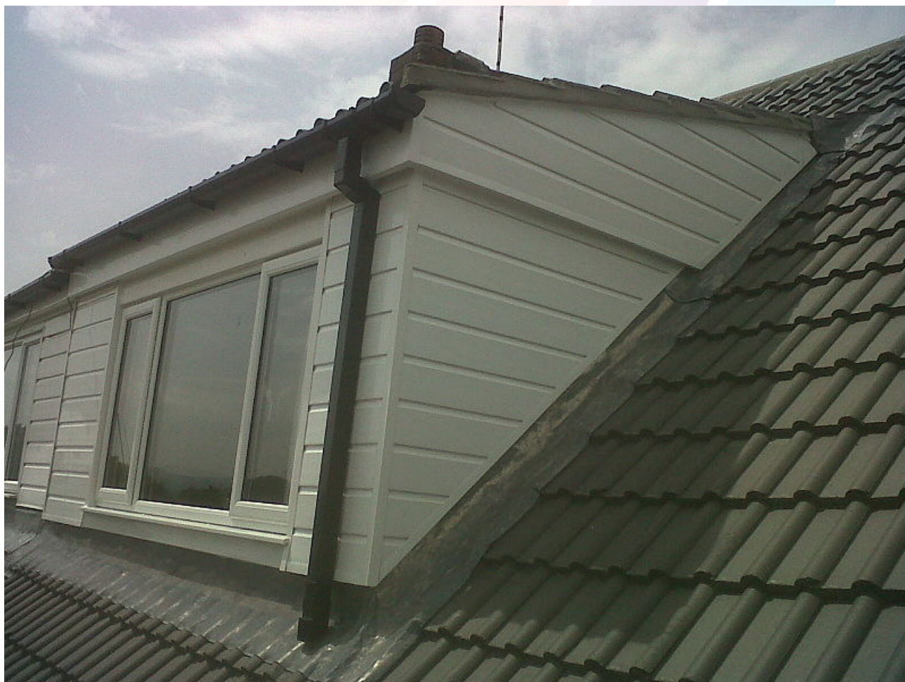
Photo: Dormer window with lead flashing. Concrete tile re-roof with UPVC dormer. Concrete tiles roof and dormer undertaken by Crown Building Services Halifax By Crownbuild https://commons.wikimedia.org/wiki/File:Concrete_tile_re-roof_with_UPVC_dormer.jpg
